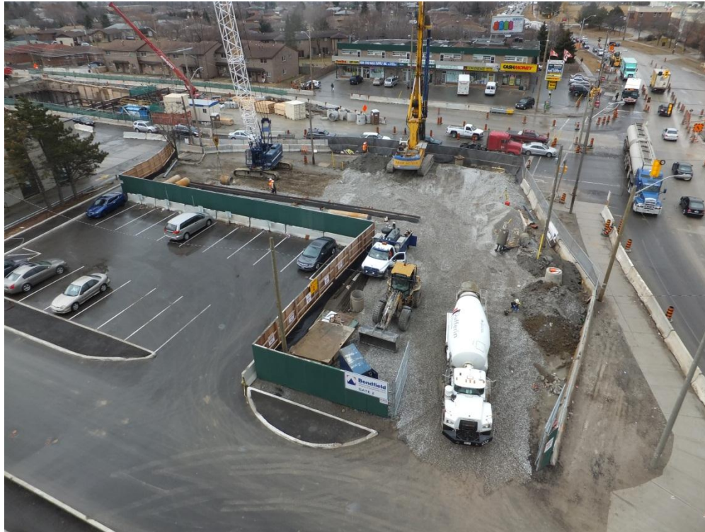
Subway construction at Keele and Finch: Just one lane each way, for multiple years.
